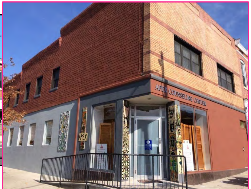
After at 3200 Eastern Avenue. Work included brick cleaning & repointing, repairs to cracks in the stucco siding, and painting.
